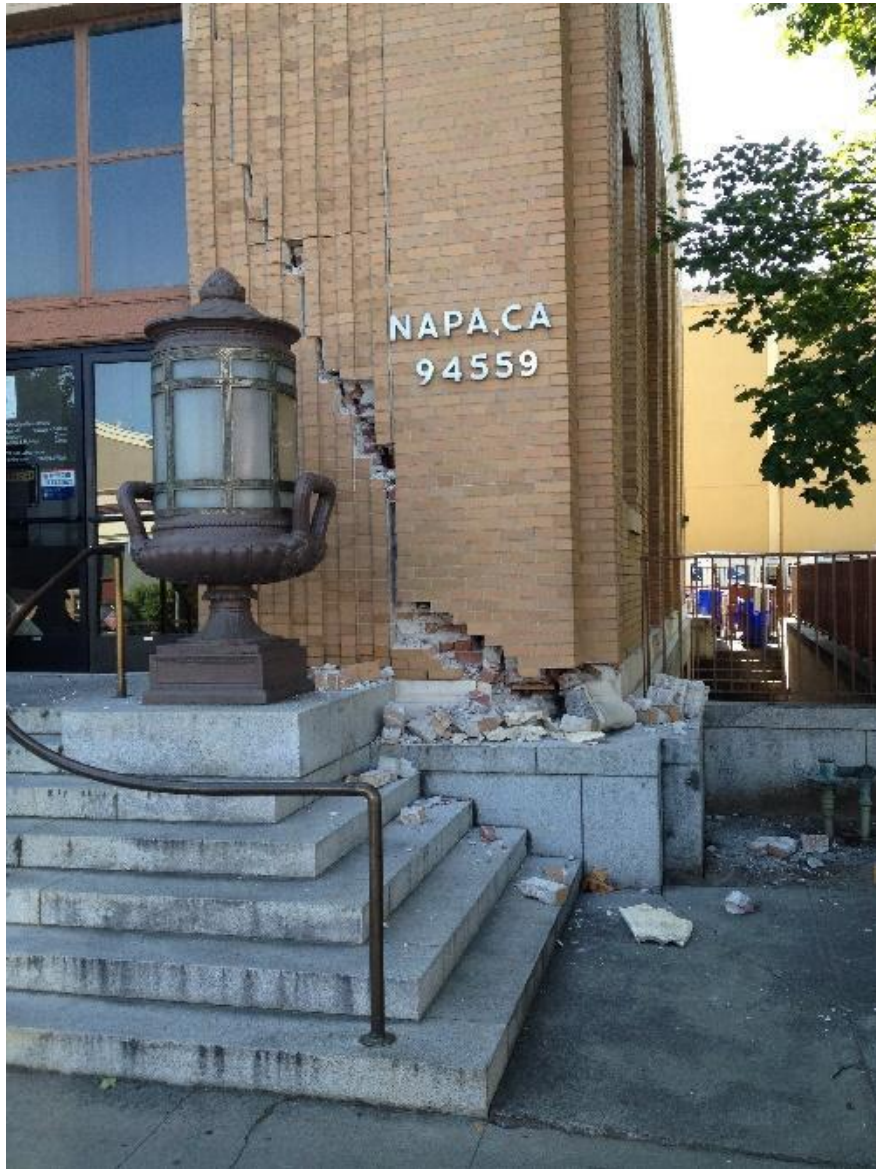
Earthquakes can cause significant building damage, especially to buildings that do not meet modern seismic safety standards.
