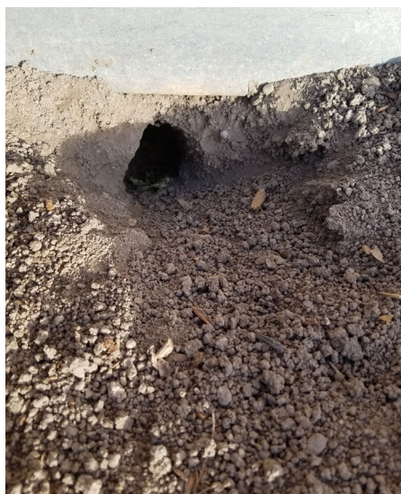
Figure 3. California ground squirrel burrow opening under structure.
