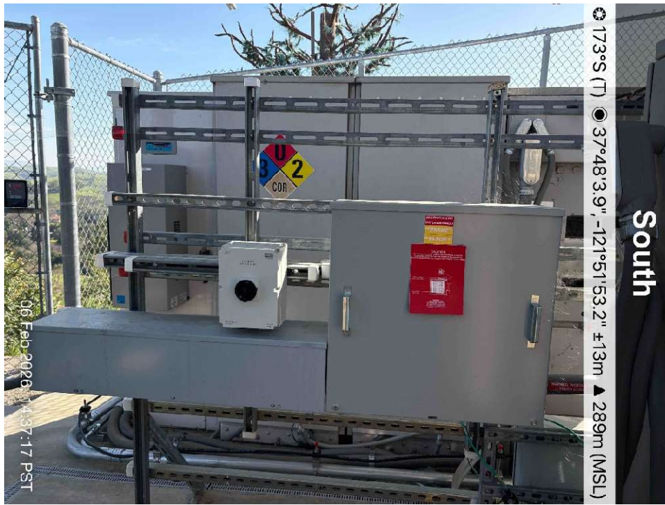
COA 19 Chainlink equipment enclosure with cabinets not exceeding fence height
