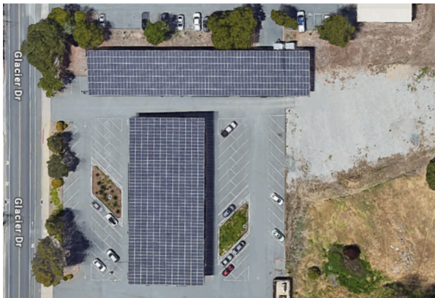
Contra Costa County’s Public Works and Sheriff’s Offices in Martinez currently have ~400 kW of solar panels on carports in the parking lots. These solar panels provide a power source for EV chargers at the parking lot as well as shade for parked vehicles
