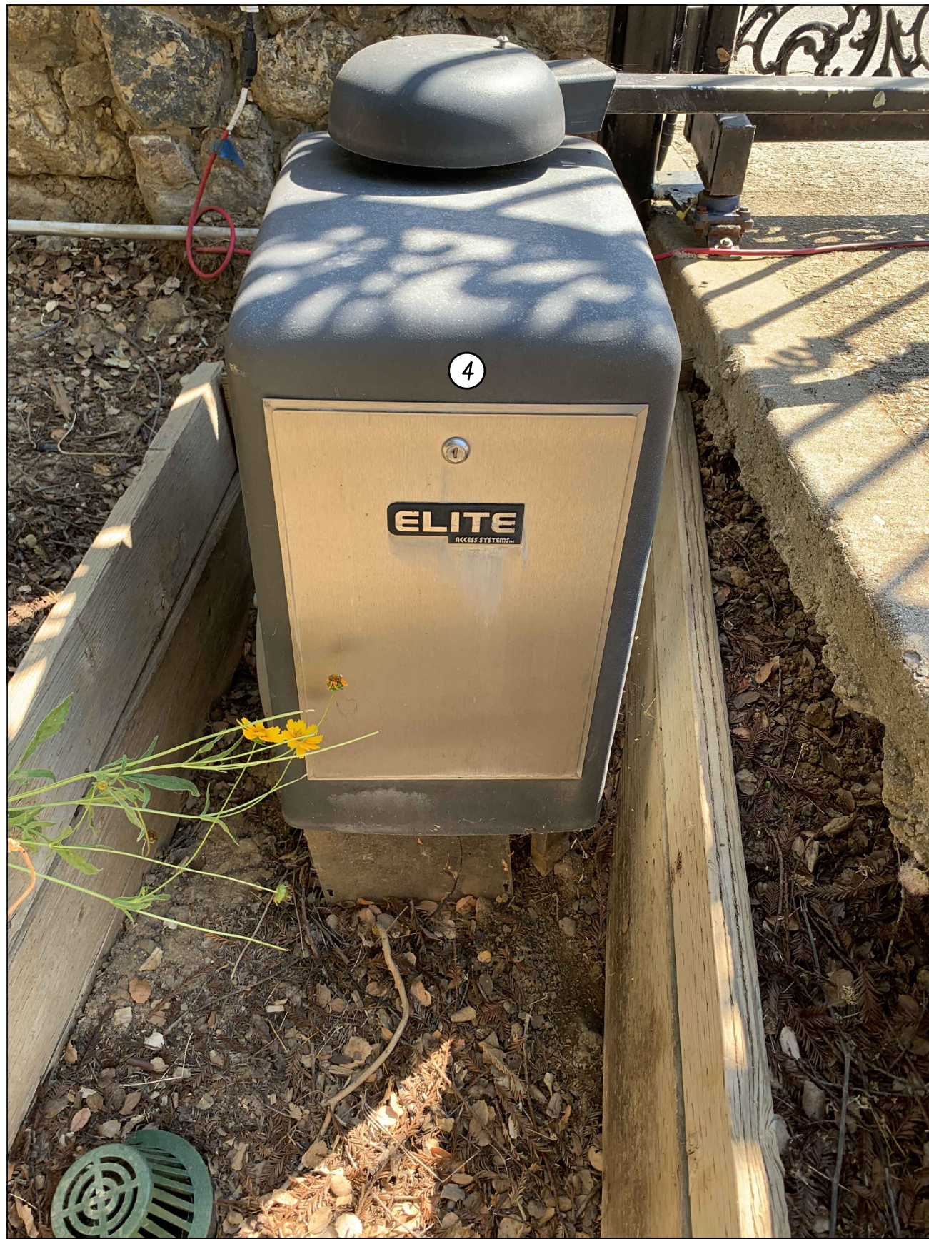
GATE CONTROLLER - NORTH SIDE SWING GATE OPERATOR
