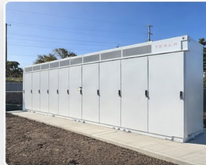
Energy Storage System
