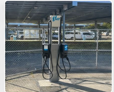
EV Charging Infrastructure
