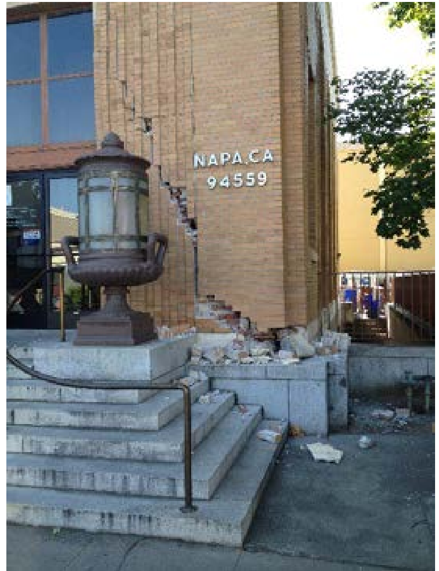
Earthquakes can cause significant building damage.
