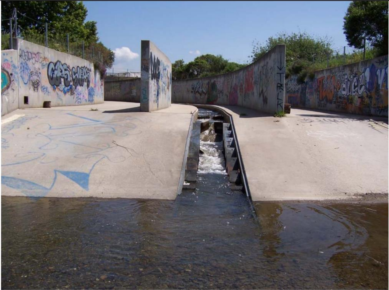
FIGURE 14: EXISTING DENIL FISH LADDER, CLEARED OF SEDIMENT, LOOKING UPSTREAM FROM SEDIMENT BASIN. PHOTO FROM EBRPD IN 2007.
