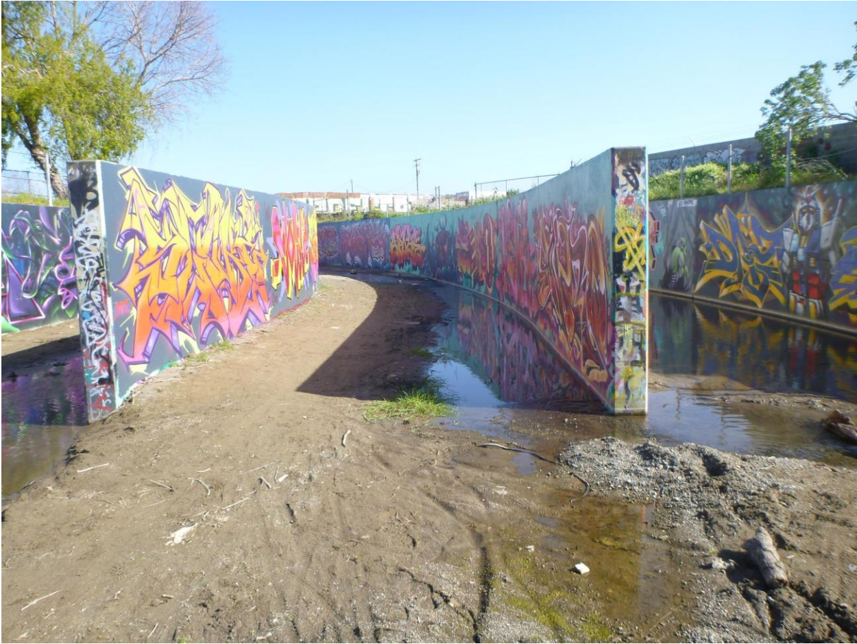
FIGURE 15: DENIL FISH LADDER, FILLED WITH SEDIMENT, LOOKING UPSTREAM FROM SEDIMENT BASIN. PHOTO FROM 2022.
