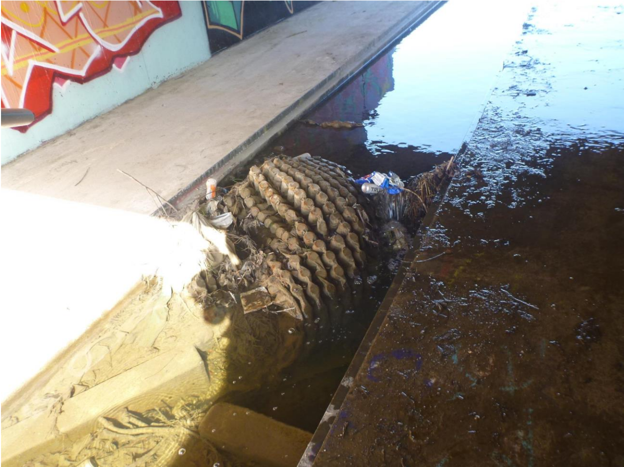
FIGURE 16: EXAMPLE PORTION OF CLOGGED WASHINGTON BAFFLES.
