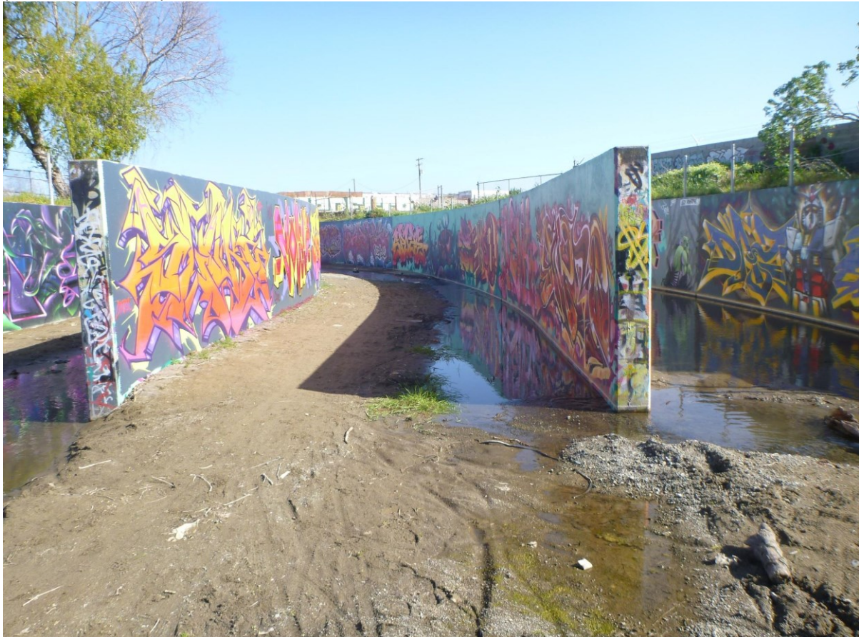
FIGURE 1 - 4: EXISTING FISH LADDER, FILLED WITH SEDIMENT, LOOKING UPSTREAM FROM SEDIMENT BASIN (PHOTO FROM 2022)
