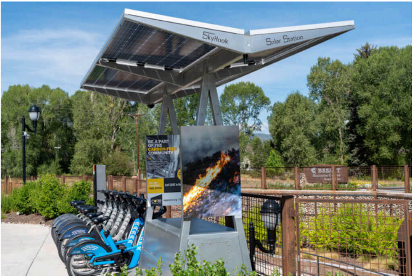
Solar e-bike charging station in Basalt, Colorado
