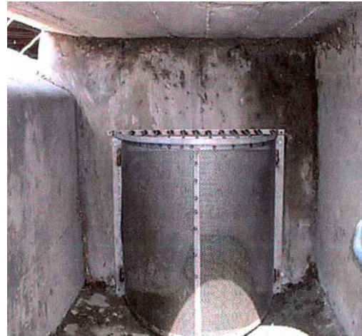
Trash Capture Device Interior
