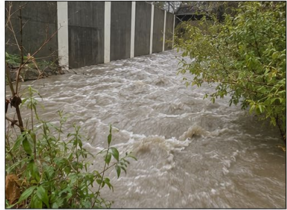
5. Water Rushing Through Headwall During Storm
