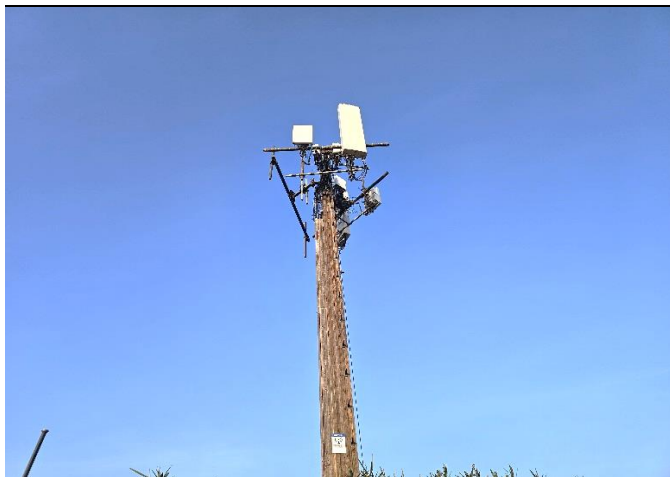
Equipment/Ground Prospective A
