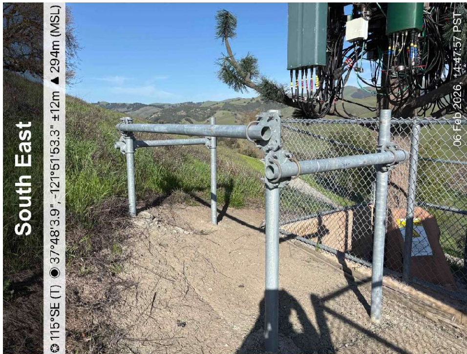
Equipment partially sunken within hillside to minimize visibility
