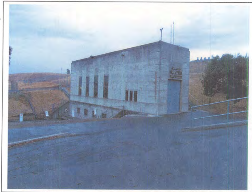
Photograph 41. Typical pumping plant on the Contra Costa Canal (Pumping Plant No. 4 shown), milepost 7.05, camera facing west, November 7, 2005.
