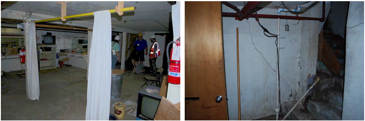
Figure 8: Basement. Left: General view. Right: Stairs up, showing cracked and buckled walls.
