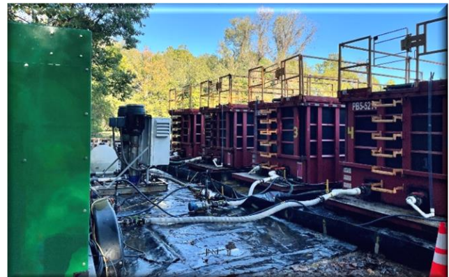
Example Bulk Mixing Tankage
